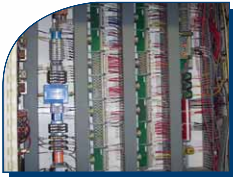
Inside of a Panel
